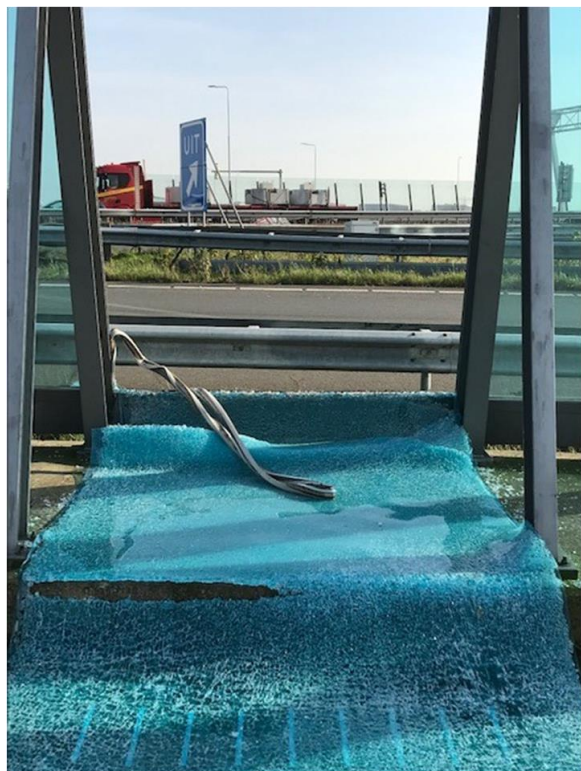
Fig. 1: Failed tempered laminated glass sound screen panel
