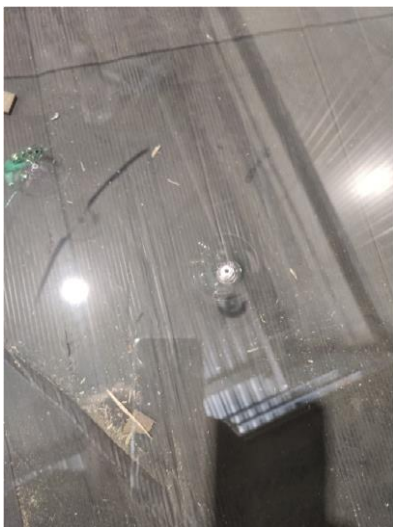
Fig. 5: Cone crack in the annealed glass after critical impact
